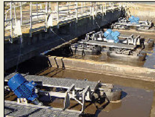
Floatation aerators at work
